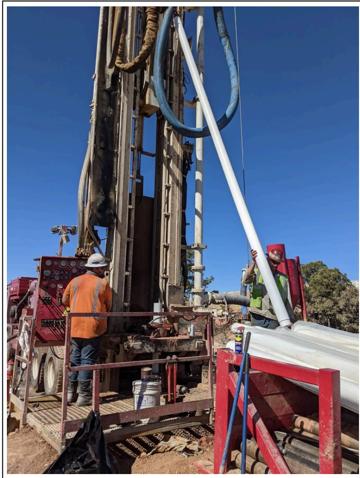
17. 2/24/2021: Major drilling 5-inch-diameter SCH 80 PVC for construction of monitor well 396-2021-02 (view to northwest)
