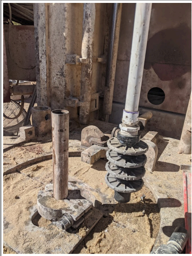
21. 3/2/2021: 1-inch-diameter tremie pipe for sand placement and PVC swab assembly to settle sand filter pack along well screen
