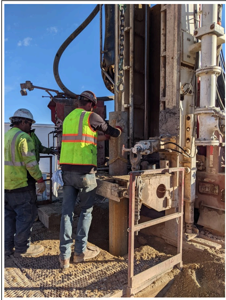
9. 2/10/2021: Major Drilling crew maneuvering surface casing into place at monitor well 455-2021-01 (view to west)
