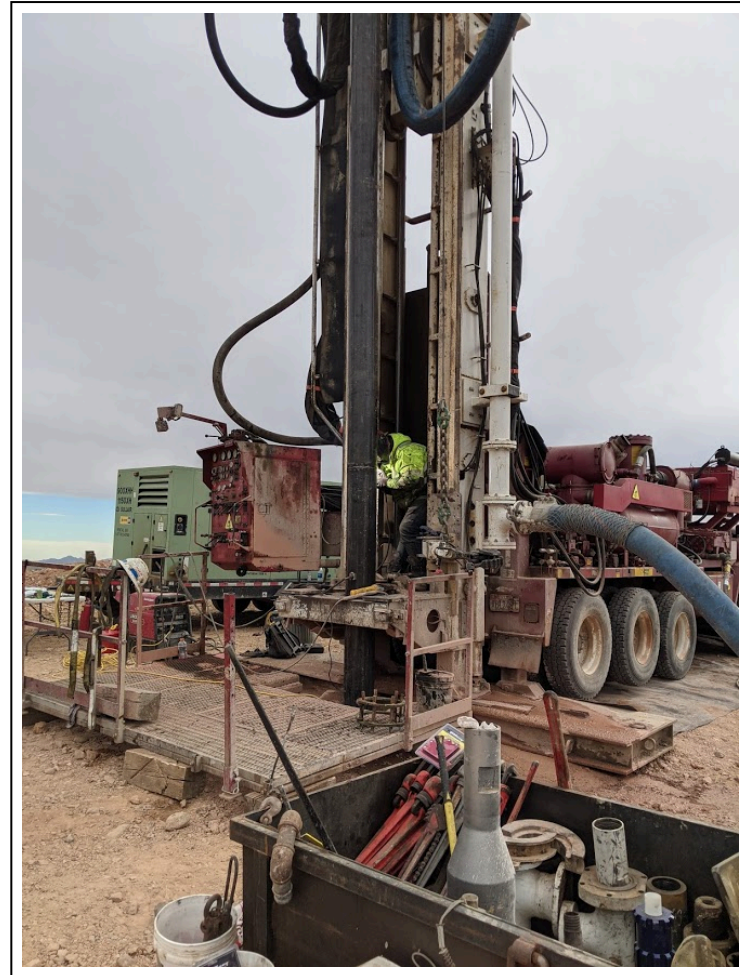
10. 2/10/2021: Major staff welding together surface casing joints at monitor well 455-2021-01 (view to southwest)
