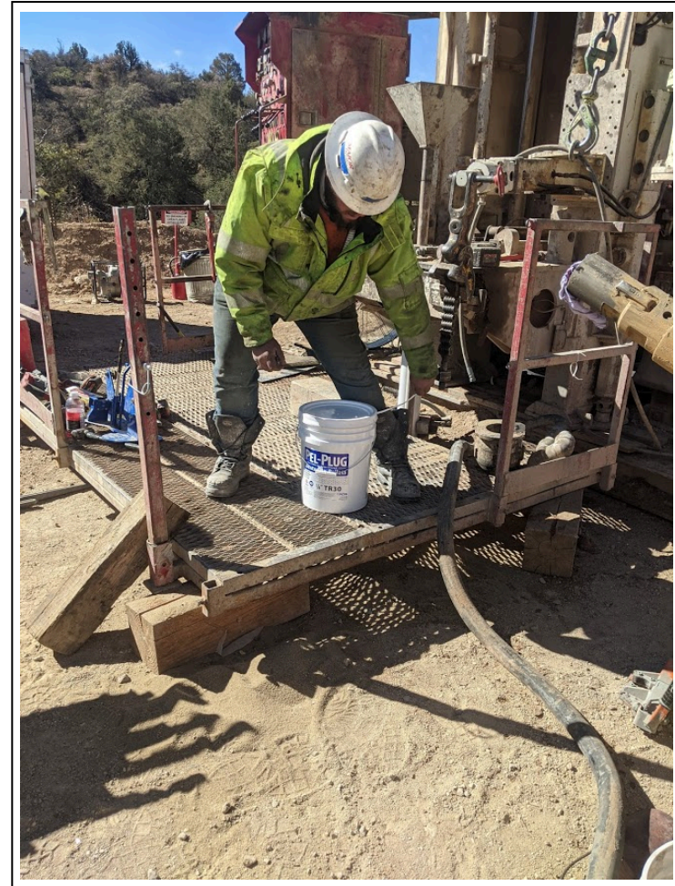
22. 3/2/2021: Major crew member opening a bucket of ¼-inch coated bentonite chips to create a seal above the filter pack at monitor well 166-2021-01 (view to southwest)
