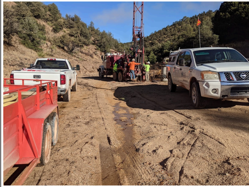
1. 12/10/2020: Enviro-Drill advancing split spoon into alluvium downgradient of Deadman Canyon system (view to north)
