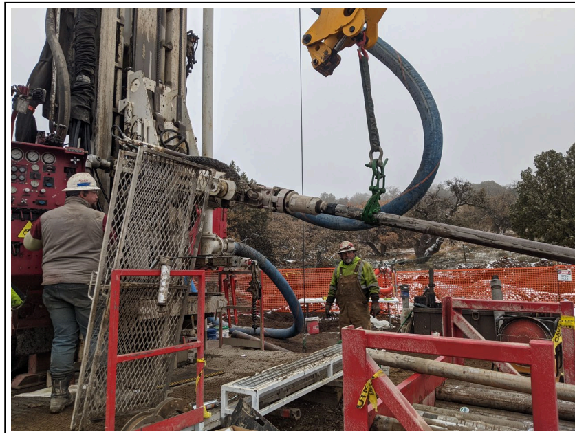
12. 1/20/2021: Crew using pipe tongs to safely maneuver drill rod into place and make connections to advance boring at 396-2021-01 (view to northeast)
