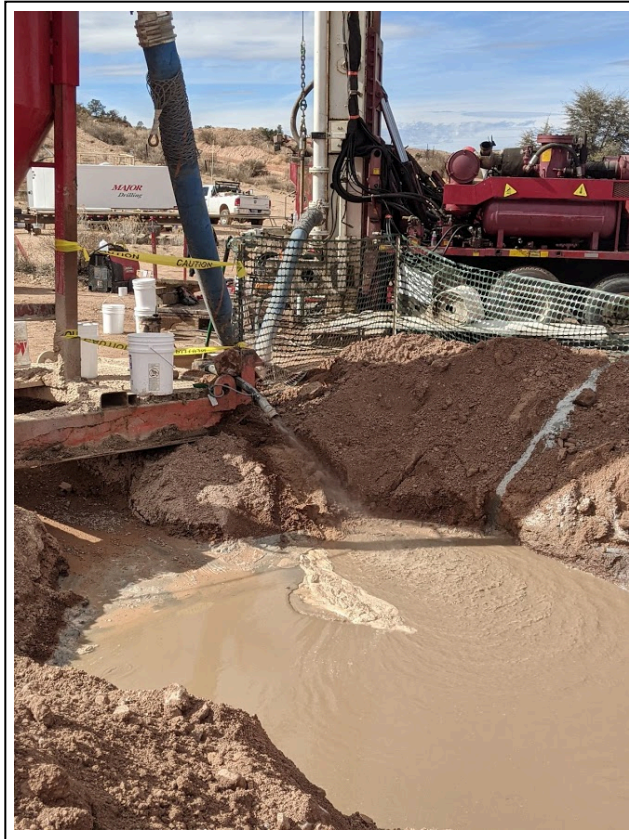
25. 2/3/2021: Development of monitor well 286-2021-01; water is airlifted from well casing and discharged to earthen sump (view to west)
