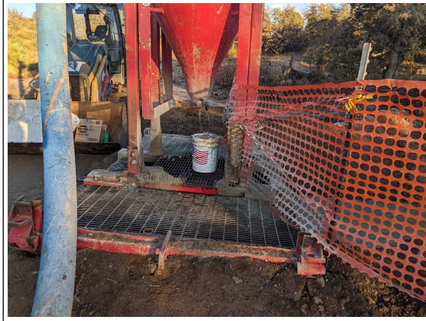
15. 1/23/2021: Water is flushed from the borehole using air pressure; this water is observed at the cyclone, and is collected in an earthen sump (view to northeast)
