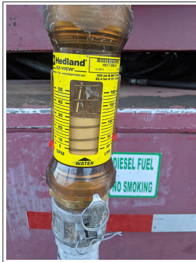
14. 2/5/2021: In-line water meter allowing drillers to monitor rate of water injection during drilling
